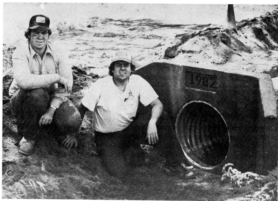
Dan Robirds and Larry Rose with PSRMA culvert No. 1,, an example of the kind of mundane work that has to be done before finish grading the sub-roadbed.
